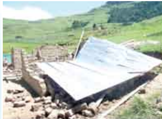
Storm damaged houses in Engcobo Local Municipality.
